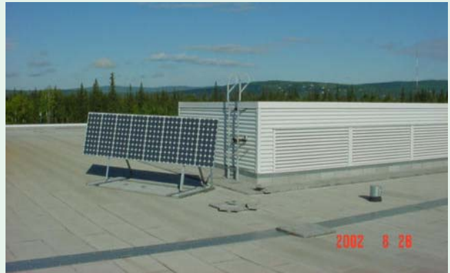
Solar panel set on Randy Smith School
